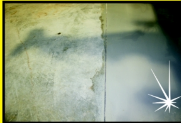
Zyrex on Right Bare Concrete on Left
