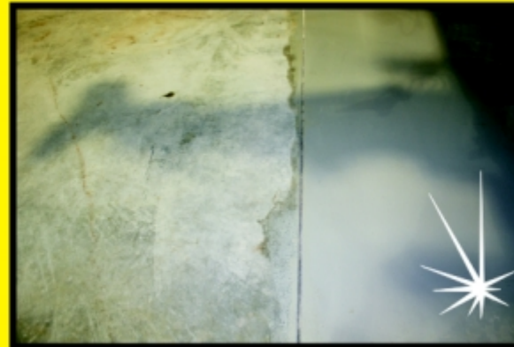
Zyrex on Right Bare Concrete on Left
